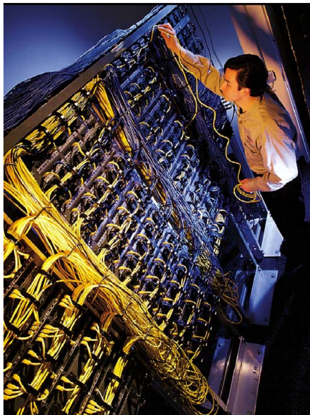
Fig. 1: iTRACS® Enabled Network Cross-connect A new set of intelligent network management tools help address Sarbanes-Oxley challenges in a manner unique from other systems.
